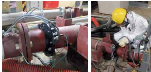
Monitoring system for pipe thickness observation
