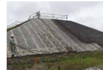
Construction of embankments utilizing the planting soil obtained by from parts of the tsunami debris.
