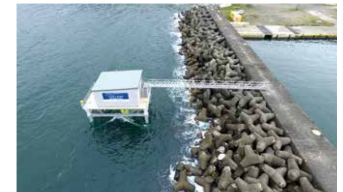
Tidal Power Plant
