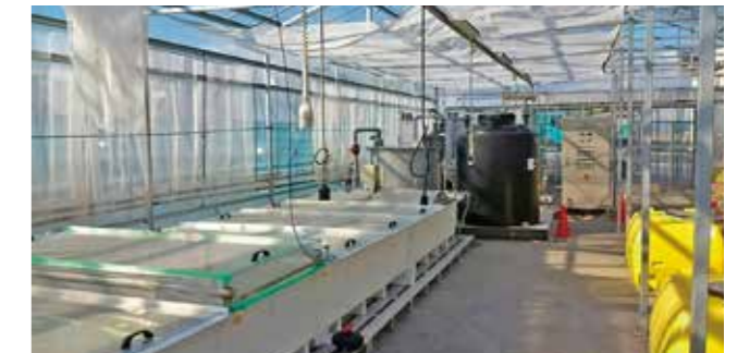
Pilot Testing Facility at the Minami Gamou Water Purification Center
